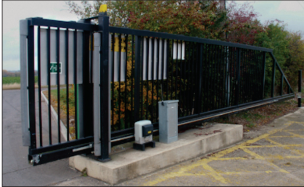
Sliding electric gates
